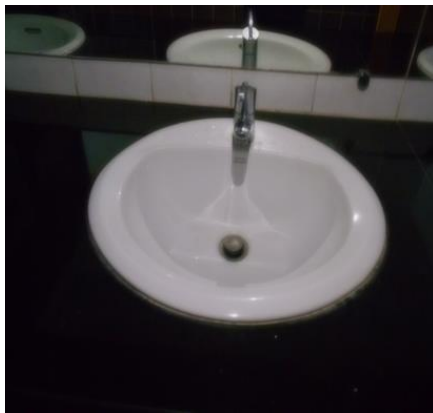
Washbasins water-saving push taps
