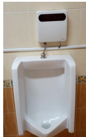
Urinals water-saving sensor
